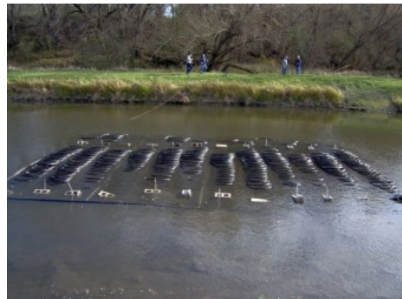
Figure 21b. Water heat exchanger using a pond (Photo: http24)
