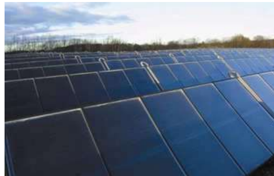
Figure 26b. Type b) Solar Thermal Collector field on the ground (Photo: ARCON/ESTIF 2016)
