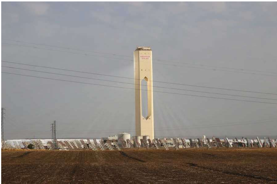
Figure 27. Solucar PS10 is the first solar thermal power plant in the world that generates electricity with this technique in a commercial way, near Seville, Spain (Photo: Naja Marot 2017)
