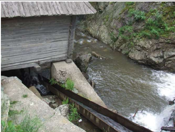
Figure 23a. Micro hydro power in Eftimie Murgu village, Caraş Severin county, Romania (Photo: Maria Bostenaru Dan 2008)
